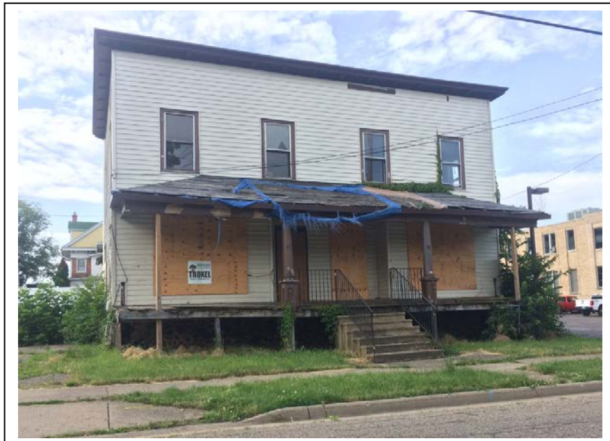
Figure 2. Picture of façade of building. Years of deferred maintenance and vacancy resulted in deterioration of the front porch, vandalism, and neglect. Picture taken by City staff on July 2, 2019.
